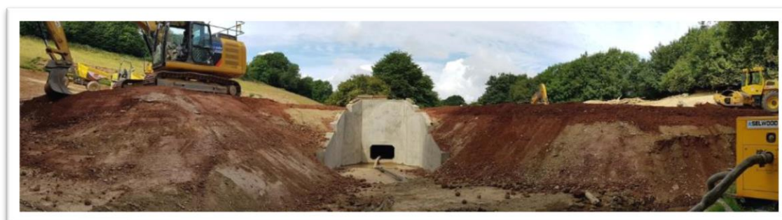
Looking south in Area 2, 2.5m tall with another 2.5m to be added to reach final crest level.
