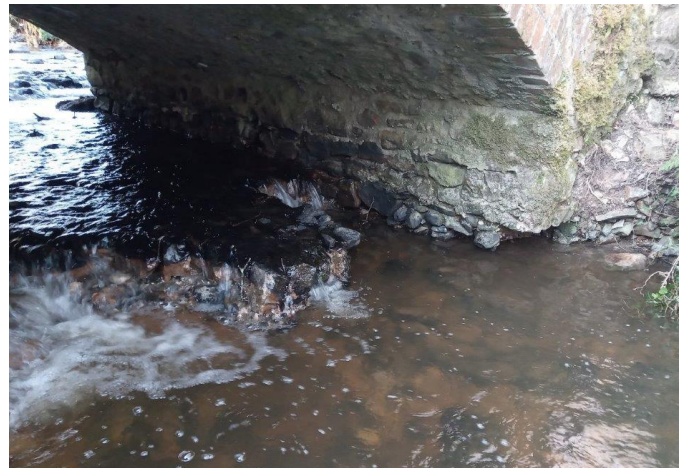
Undermined bridge in need of repair
