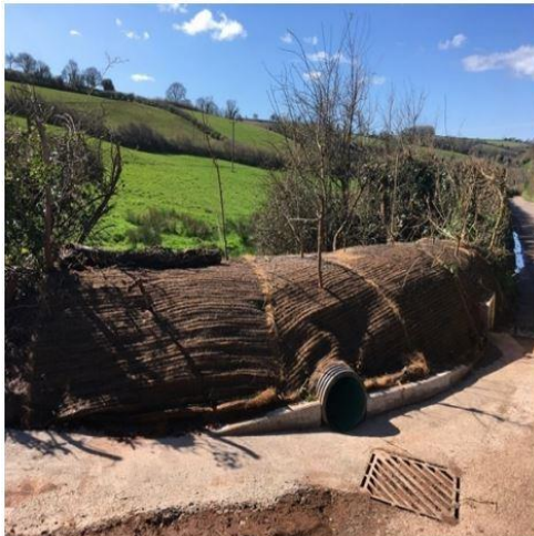
New buddle holes installed on a key surface water flow path into the village.
