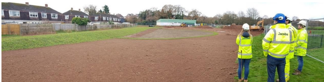
Photo taken of the new flood bund and flood attenuation area prior to seeding of the area.
