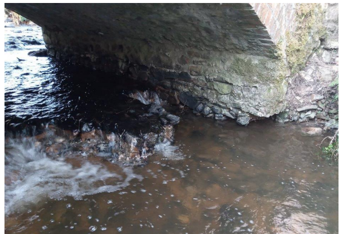
Undermined bridge in need of repair
